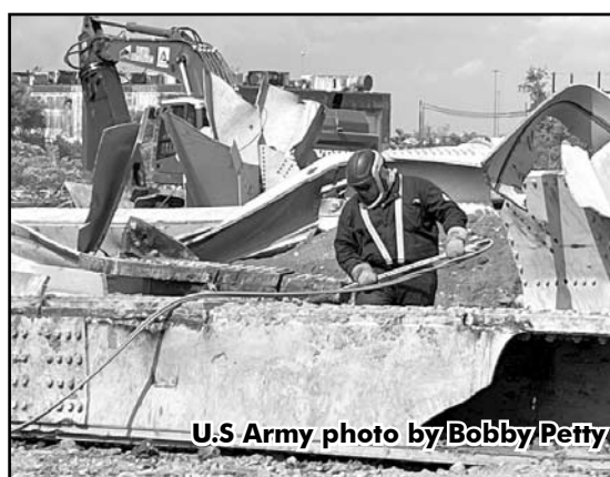
TORCH & Armed with oxyacetylene torches and a CLAW claw excavator June 5, 2024, at Sparrows Point, Md., Unified Command salvage workers carve up a section of steel truss removed from the Fort McHenry Federal Channel near Francis Scott Key Bridge
