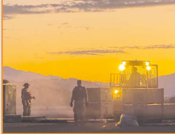
STORM CROW: Airmen prepare to build tents during Storm Crow at Fort Hunter Liggett in California, June 24. The exercise is designed to demonstrate readiness to conduct air base opening missions in contested environments. U.S. Air Force photo by Staff Sgt. Scott Warner
