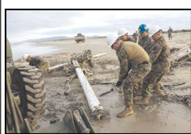
BOAT RESCUE Marines with 7th Engineer Support Battalion, 1st Marine Logistics Group, remove debris from White Beach at Camp Pendleton Aug. 23, 2024. 7th ESB provides mobility, countermobility, survivability, general engineering, and explosive ordnance disposal support to I Marine Expeditionary Force. U.S. Marine Corps photo by Lance Cpl. Jeslianne A. Torres
