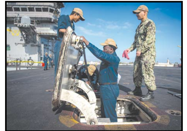
TOPSIDE WORK Sailors conduct preventative maintenance on the flight deck aboard Nimitz-class aircraft carrier USS Carl Vinson Aug. 22, 2024. Vinson is currently pier-side in its homeport on Naval Station North Island San Diego. U.S. Navy photo by MCSN Kenneth Ostas
